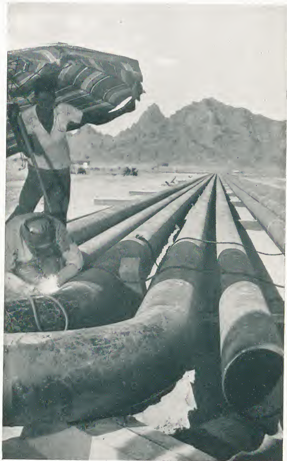
'S & L' steel pipes being laid between the harbour and the Aden refinery of the Anglo-Iranian Oil Co.
